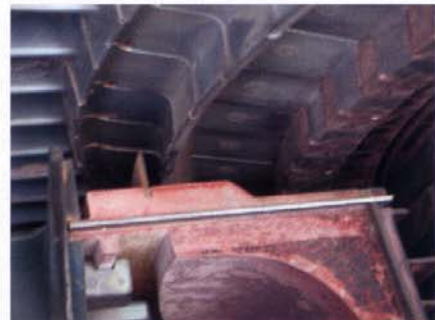
2-3. Dimensional checks pinpoint deformation and other problems that should be addressed in your repair spec (below)
